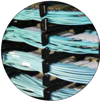
Front cable management
