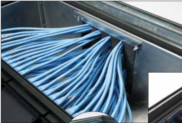
Firestop block adds protection to network wiring.
